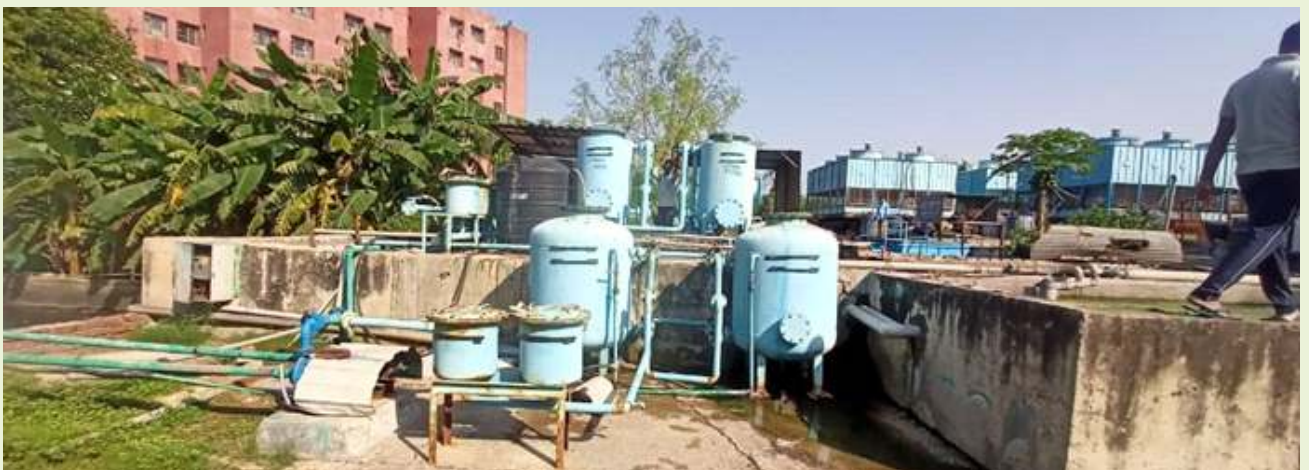
PREVENTING WATER SYSTEM POLLUTION
